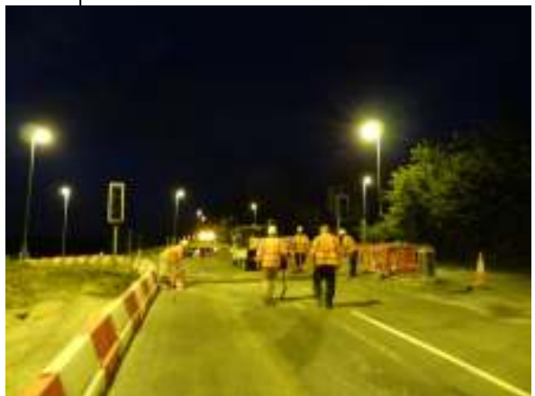
The crossroads has new traffic lights installed – at night Photo Geoff Watkins
